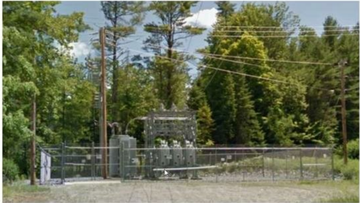
Typical Substation at point of interconnect – located on site adjacent to transmission line
